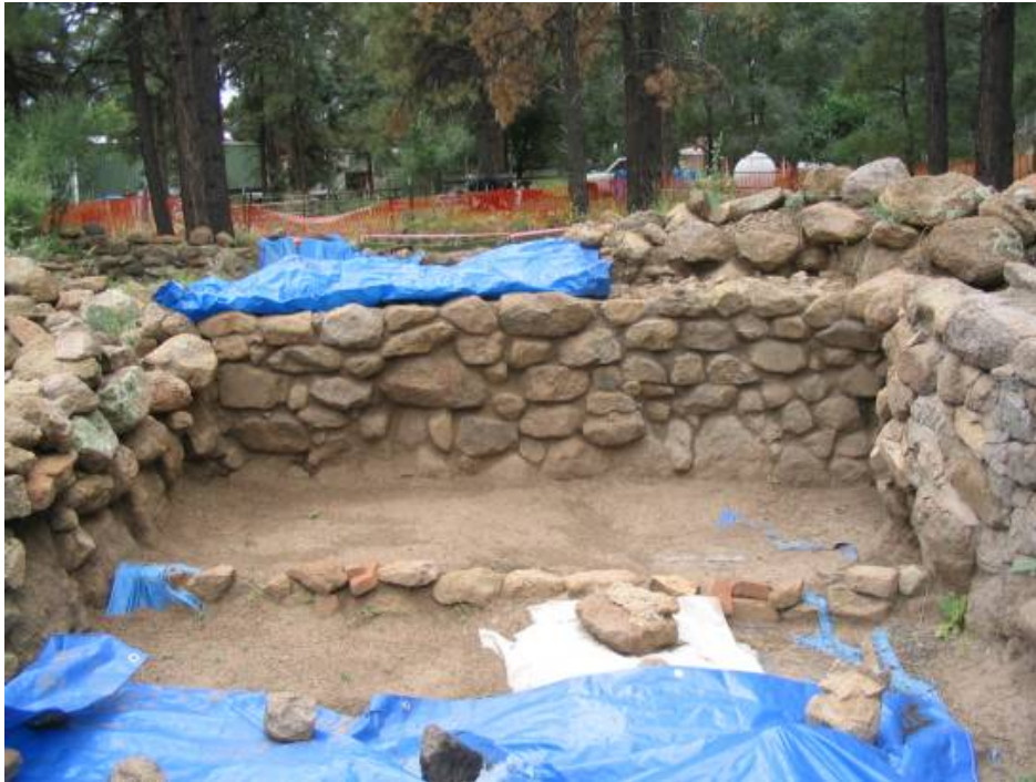
This is a photo of Room 1, south interior after stabilization has been completed this year. This work was an emergency project due to the collapse of the wall after re-excavation in 2002.
